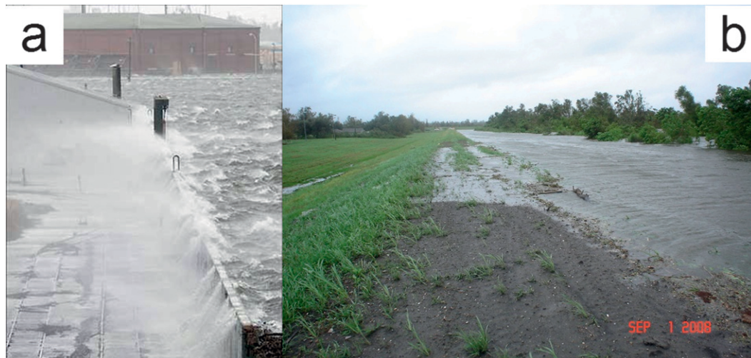
FIG. 2. Photographs during Gustav of (a) waves overtopping the IHNC walls near the Ninth Ward and (b) surge overtopping the earthen levee near Braithwaite. (Courtesy of Nancy Powell, USACE.)
